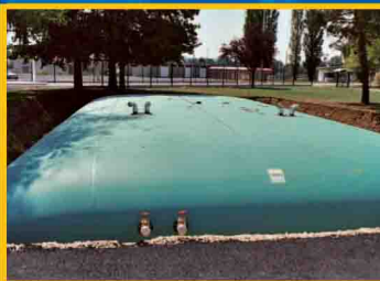
▪ Mud storage tank
