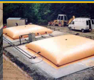
▪ Rainwater recovery tank
